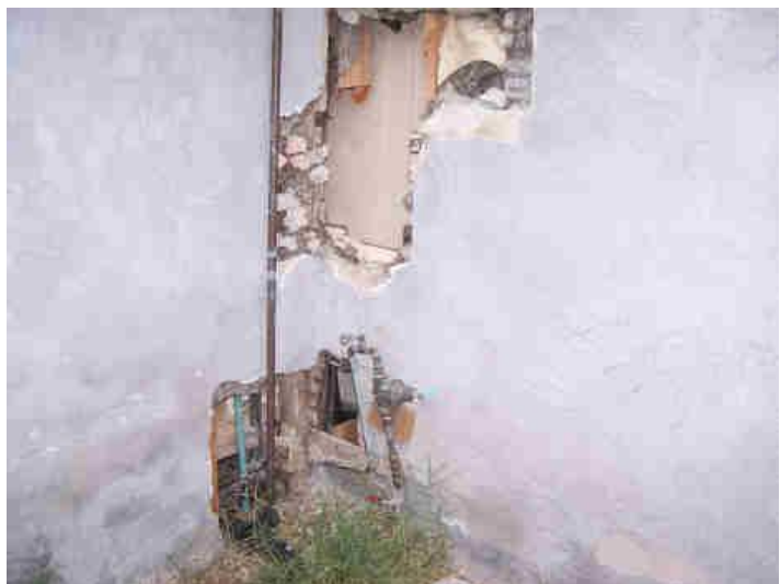
HOLES IN REAR OF SUBJECT AND UTILITY SHED
