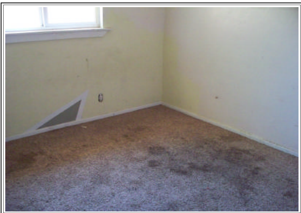
Bedroom and Stained flooring
