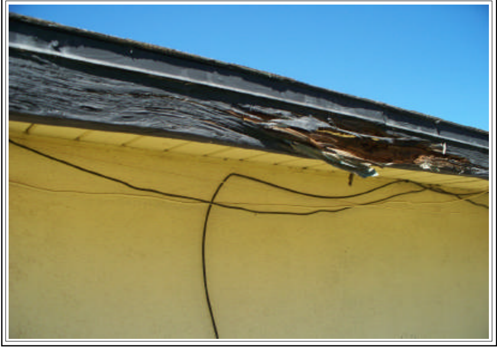
Dry rot on eaves
