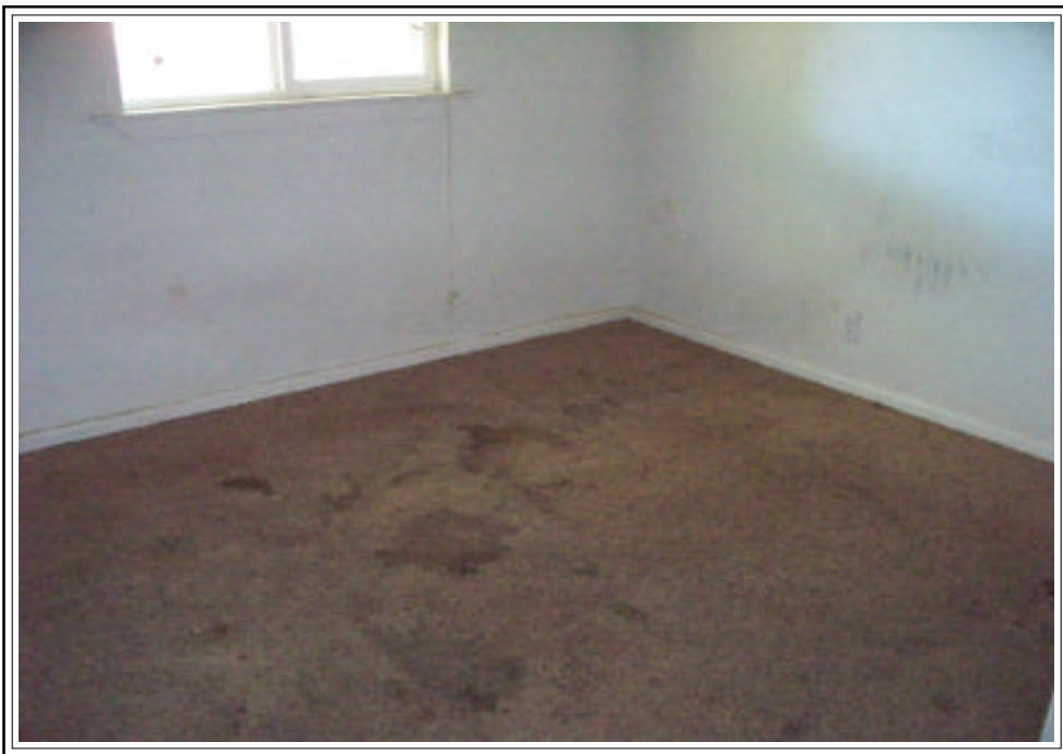
Bedroom and Stained flooring
