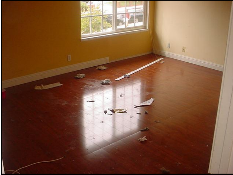
Subject Bedroom (Damaged Baseboard)
