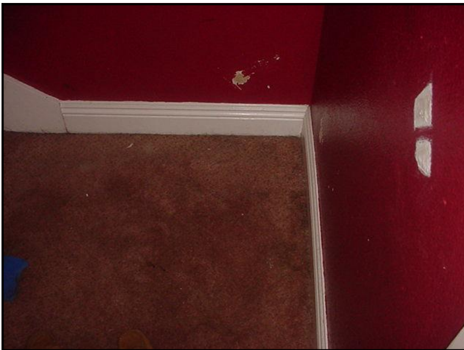
Soiled Carpet/Wall Damage
