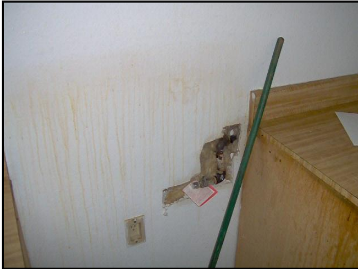
Drywall hole for Gas Line
