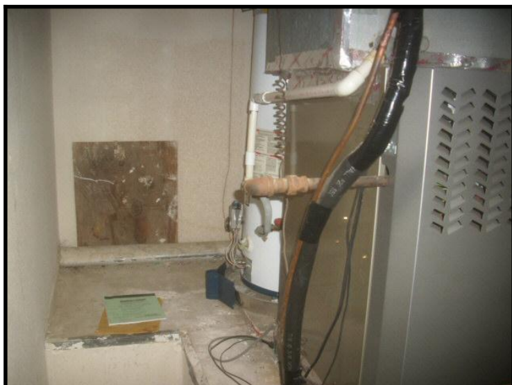
FURNACE AND HOT WATER HEATER
