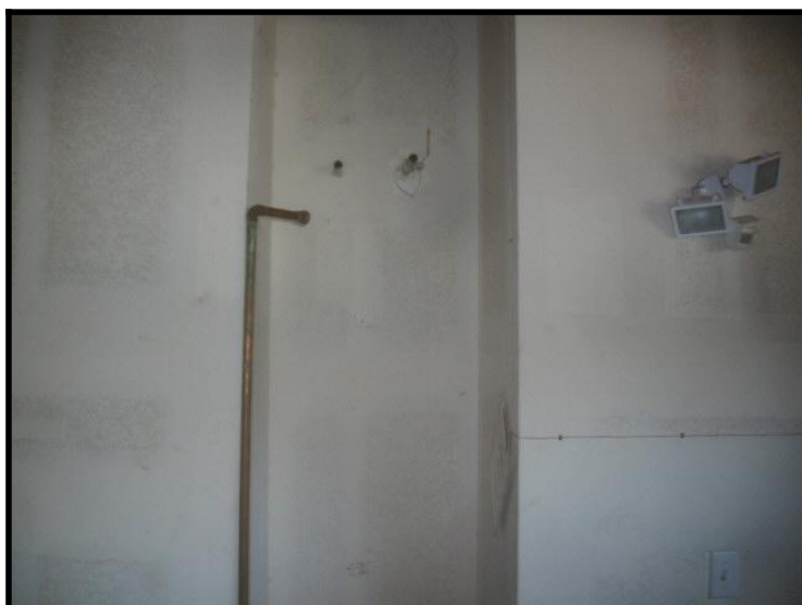
NO HOT WATER HEATER
