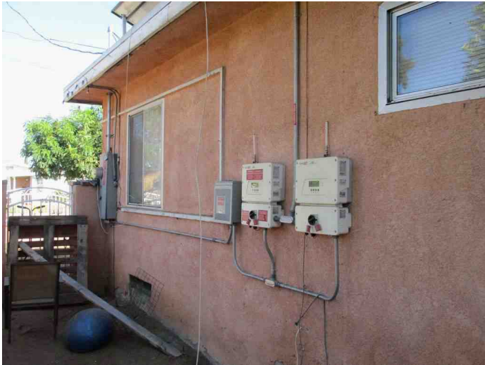
Solar Inverters / Electricity Meter
