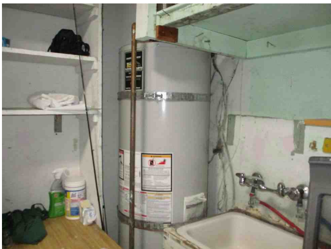
Water Heater (Strapped)
