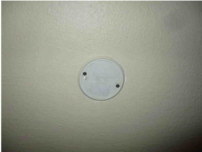
Missing Smoke/CO Alarm in Bedrooms
